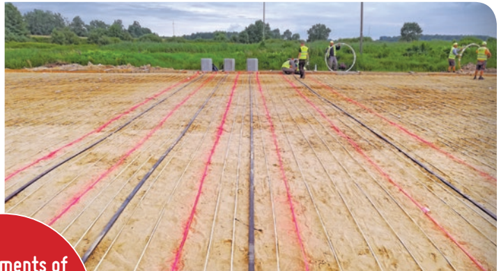
Application of 3DSensor in a road embankment
